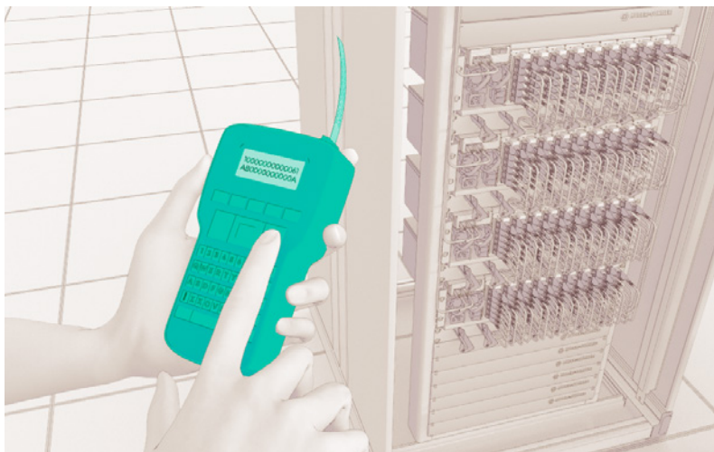
Implementation team generates installation documentation and ensures every component is labelled
